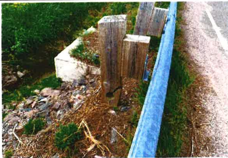
Photo Description Broken guide rail post - southwest quadrant.
